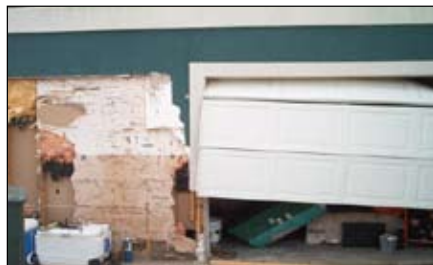
2. GARAGE DOOR FAILURE DUE TO HYDROSTATIC PRESSURE
