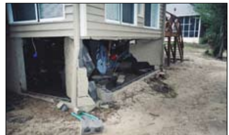
3. NON COMPLIANT FLOOD VENTS PROVIDE INADEQUATE PROTECTION, LEADING TO STRUCTURAL DAMAGE
