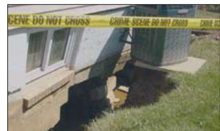
6. HYDROSTATIC PRESSURE COLLAPSES FOUNDATION WALL
