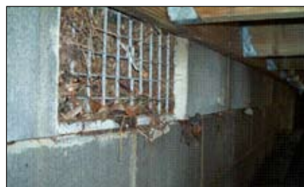
5. TYPICAL AIR VENTS CLOG WITH DEBRIS
